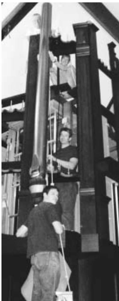
From the top: Rick Isaacs, Patrick Fischer, Andrew Gingery, and Nick Tyner hoist a pipe into place for Opus 123 in Chicago.
